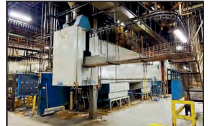
TEK-MOR 7-STAGE IRON PHOSPHATE WASH
