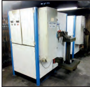
(2) NORTH AMERICAN RECTIFIER 6PF-F 12,000 AMP RECTIFIERS
