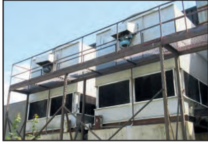
(2) EVAPCO COOLING TOWERS
