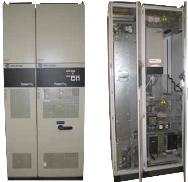
Active Front End with an IP21/NEMA 1 Rittal enclosure
