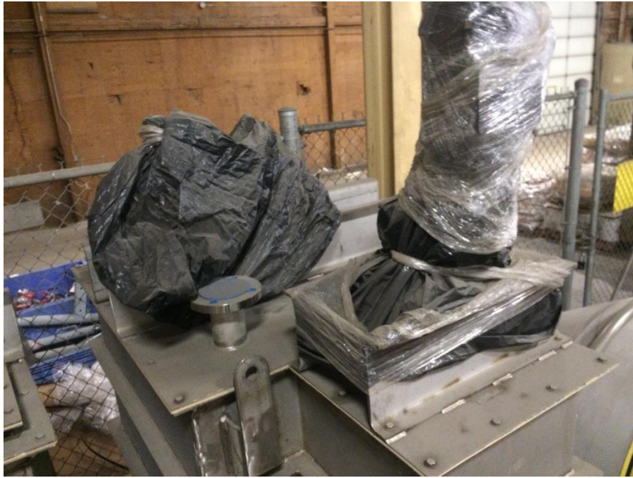
Figure 3. Photograph of the top of the flocculation mix tank, highlighting the installed agitator gearboxes and motors (covered in plastic)
