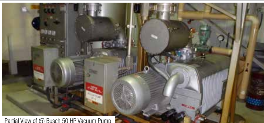
Partial View of (5) Busch 50 HP Vacuum Pump
