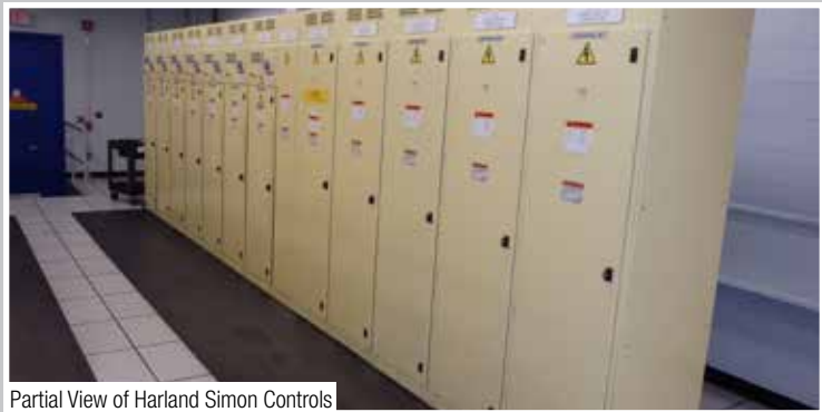
Partial View of Harland Simon Controls
