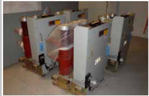
Partial View of Tech Cable and Spare High Voltage Switch Gear
