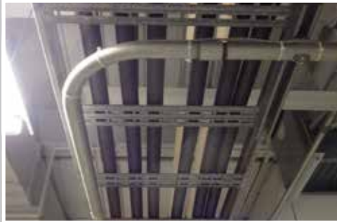
Partial View of Tech Cable and Spare High Voltage Switch Gear
